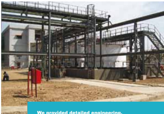
We provided detailed engineering, procurement assistance, construction and project management, and safety monitoring for the rubber chemical manufacturing facility in the state of Gujarat.
