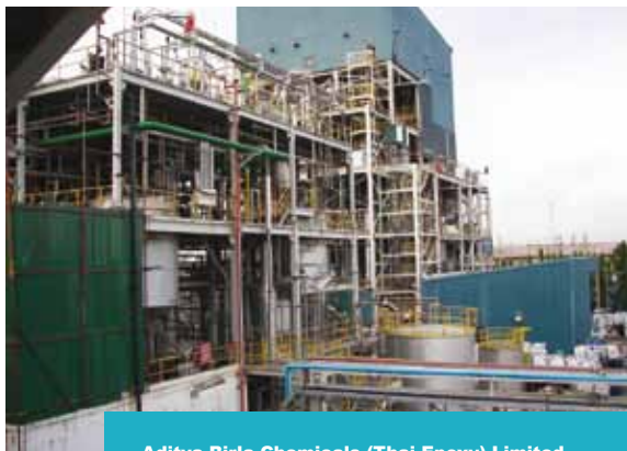
Aditya Birla Chemicals (Thai Epoxy) Limited is located at Maptaphut Industrial Estate, Rayong, Thailand. We used Plant Design Management System (PDMS) to provide total engineering solutions. This process was scaled up from research and development to pilot plant data.
